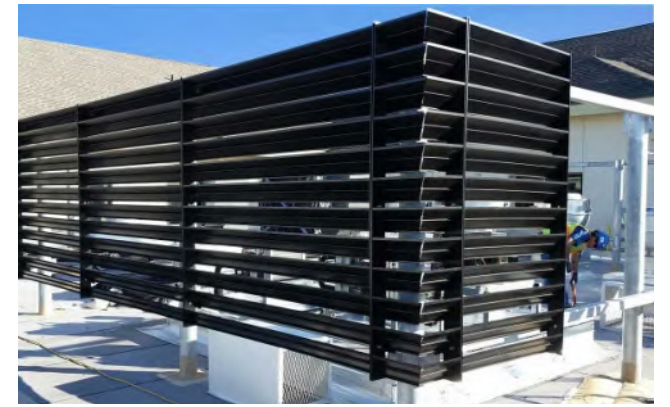
Rooftop Screening | Sharchs
