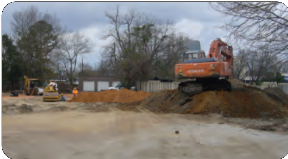
Construction is under way on the new Florence Little Theatre Complex on Dargan Street.
