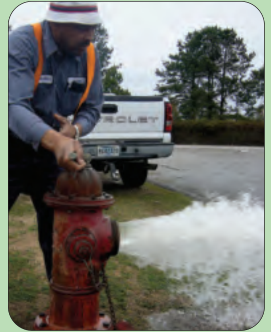
A City water production operator properly flushes a hydrant.
