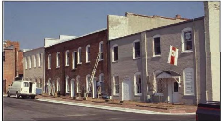
These historic buildings were renovated to include rear entries and an attractive sidewalk.
